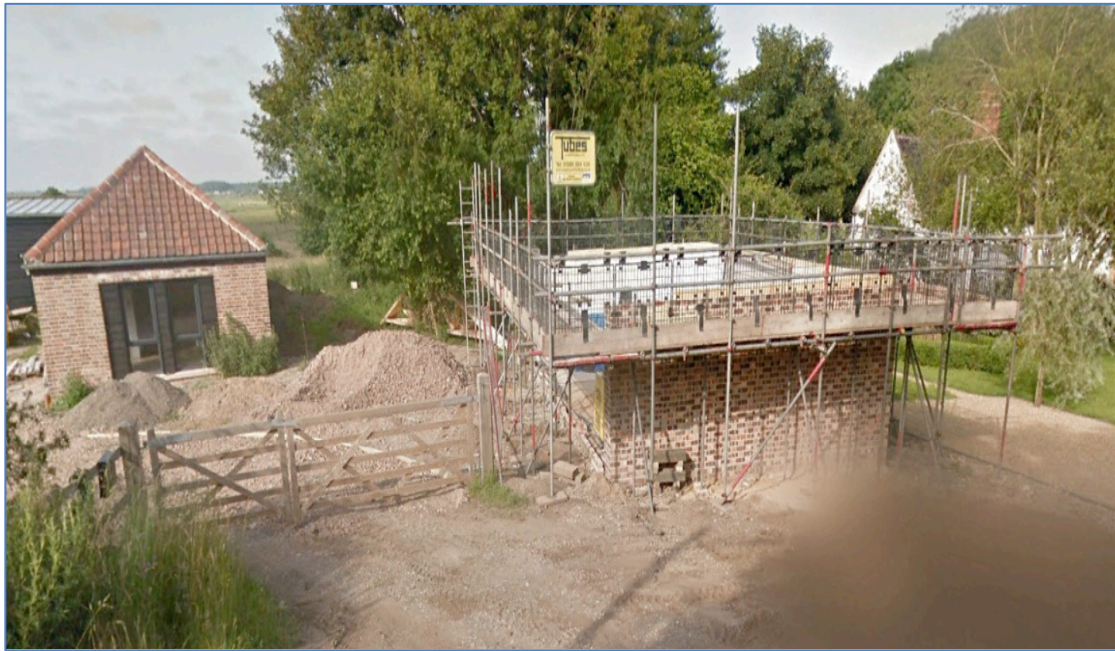
Figure 12.31: View from direction of PDA showing White House Farm to right and new development adjoining curtilage to the west © Google Earth
